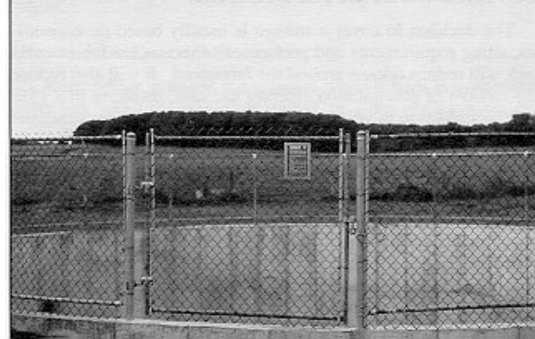
Figure 11. A concrete liquid manure storage tank with chain link safety fence. (After Hilborn, 1997).
